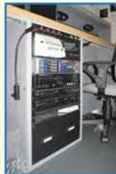
Rack Mount Equipment Suite
