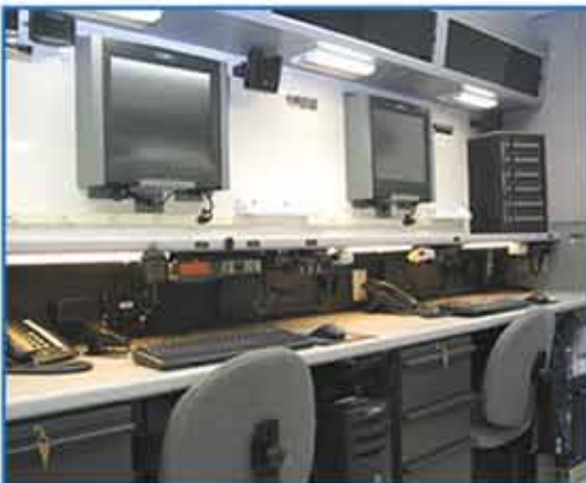
Full Communications Availability via Police Radio, Land Line Phone, Cellular, Satellite and Internet Access.
