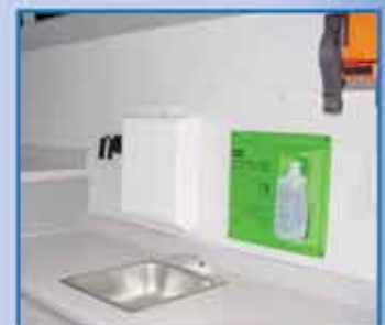
Sink and Eye Wash Station
